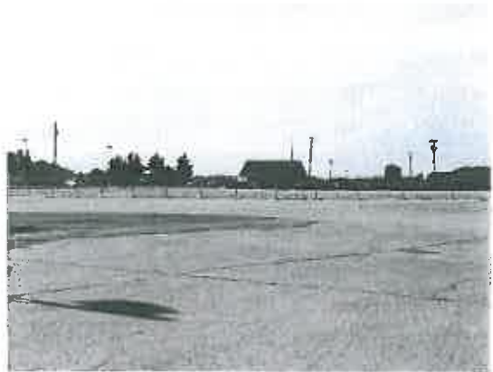
Current Strack & Van Til Grocery Store- Demolition Work on 133rd Avenue within Lincoln Plaza Shopping Center
